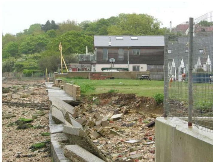
Above: Coastal erosion and defence failure at Gurnard Luck, May 2009
